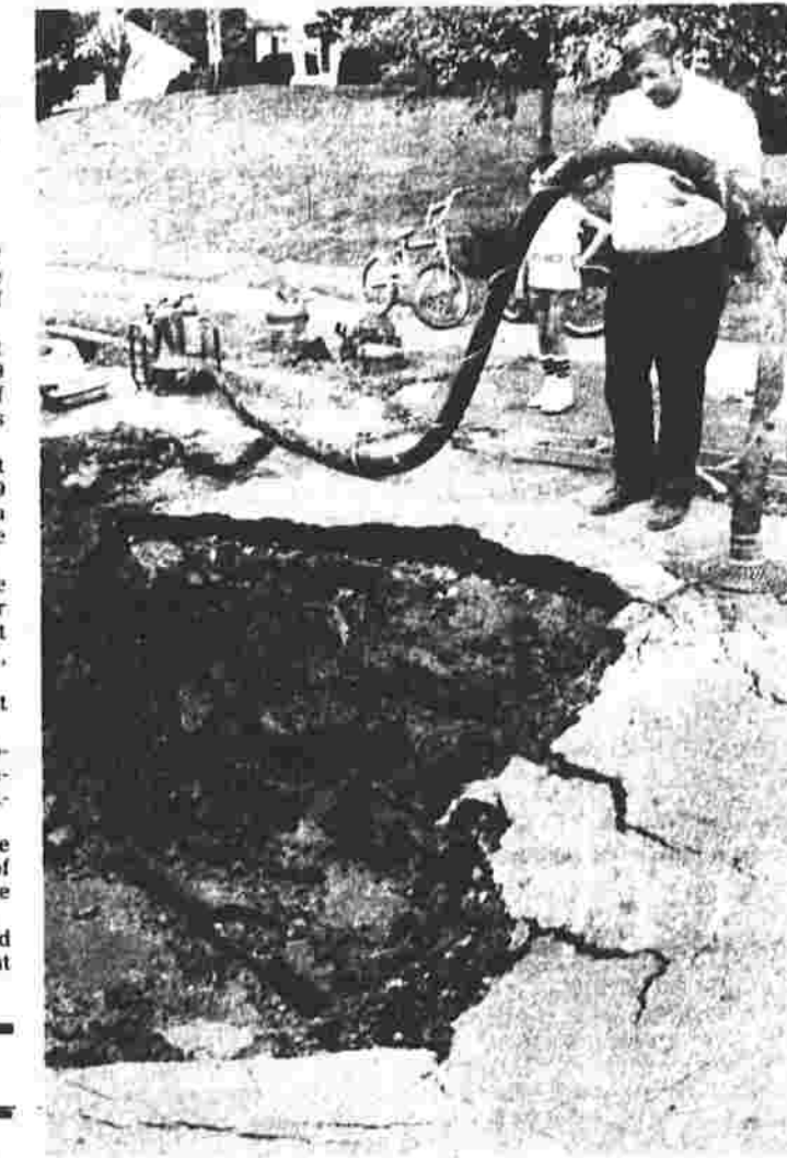
Town workers dig around a broken water main on Nutmeg Drive this morning that caused a portion of the street to collapse. The cave-in left a 15-by-6 foot hole in front of a house at 89 Nutmeg Drive.
